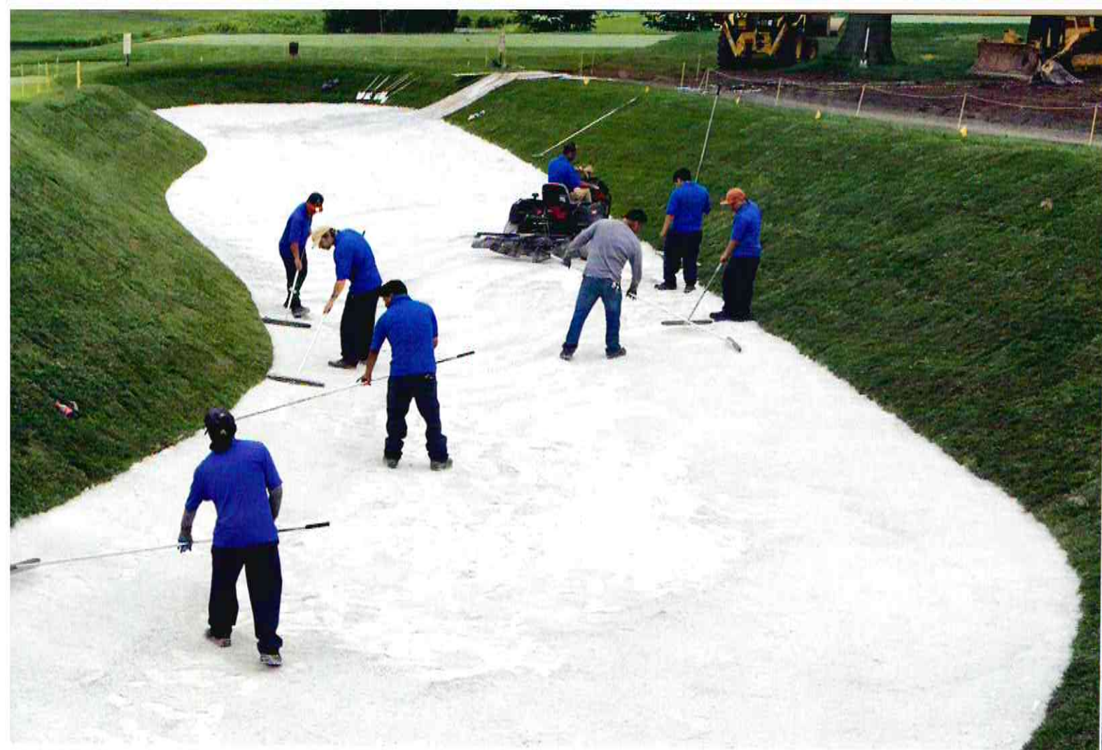
ABOVE: Hackensack's crew works to restore the back bunker on the par 3 12th hole, the Redan.
